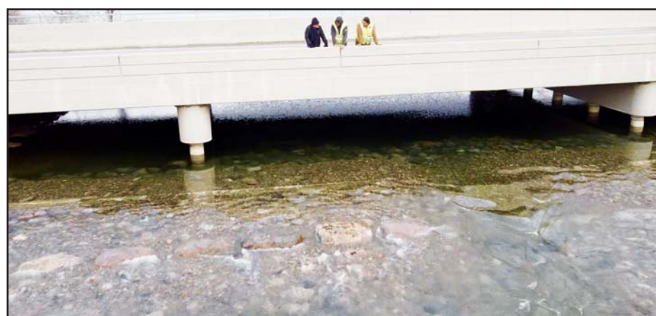
Otter Tail Lake Outlet Dam and Rock Ramp, December 2023 (Photo by Tom Kuder)
